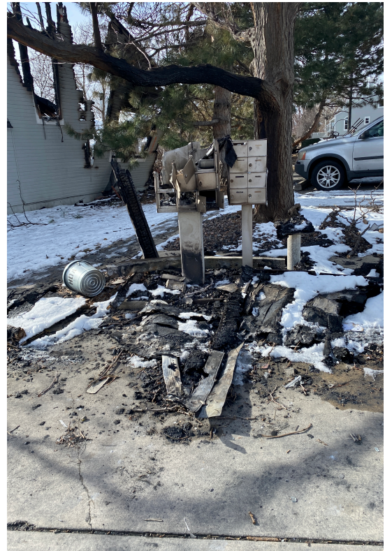
The fire was hot enough in places to melt the metal mail boxes. Here’s a photo I took of a partially melted collection of boxes at a nearby condominium complex.
